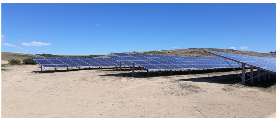
Fig. 3.2 Images from solar panels installed in Madanaj, Gjakovë
