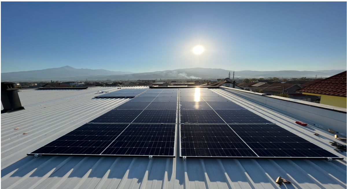
Fig . 3. 3 View from the realization of a generator for self-consumption of a 7 Kw, individual.
