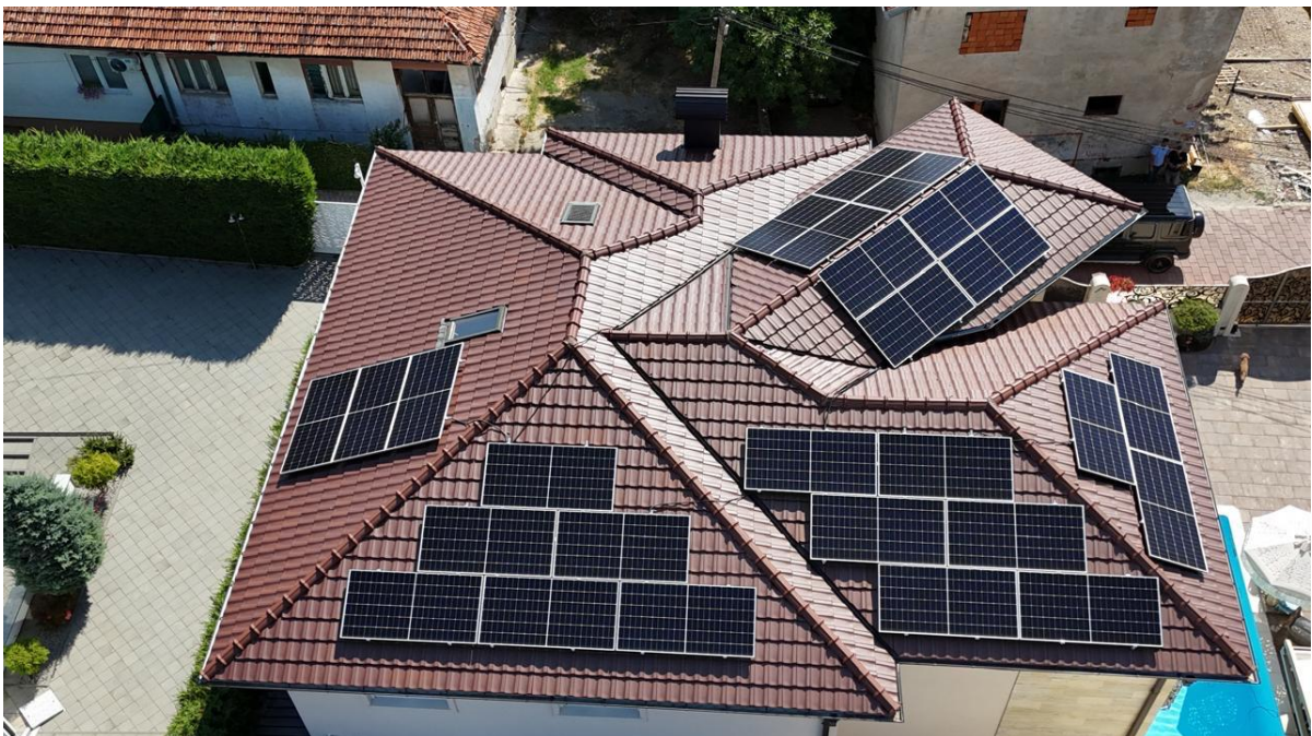
Fig . 3. 3 View from the realization of a generator for self-consumption, natural person, 7 kW
